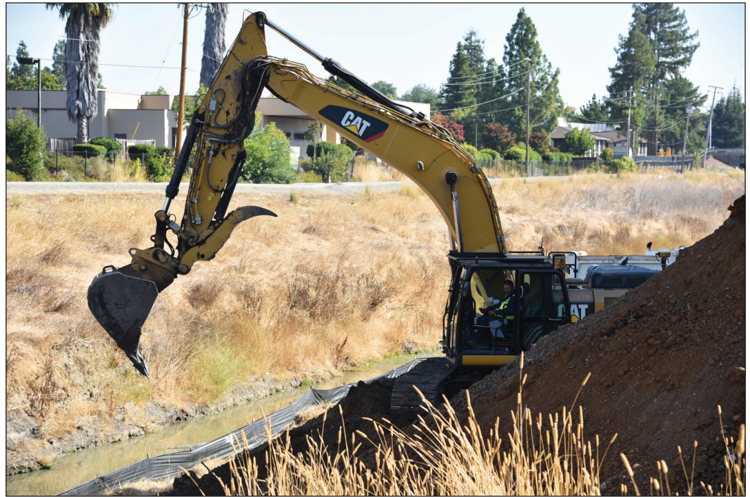
Repairs are underway by the Corps' San Francisco District to a levee damaged by winter storms in Pleasanton.
